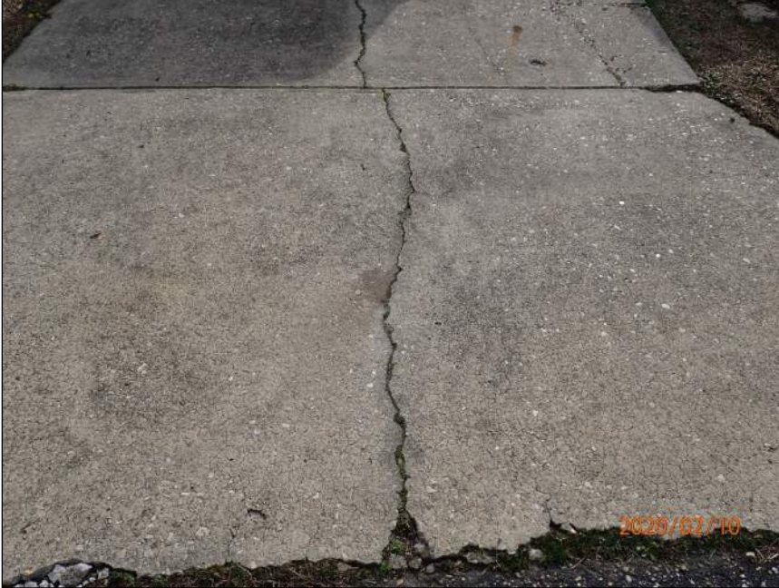
Photo 5 Cracks in concrete driveway
