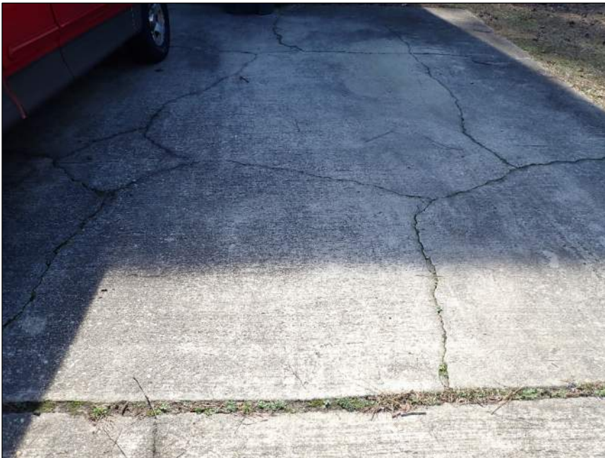
Photo 6 Cracks in concrete driveway
