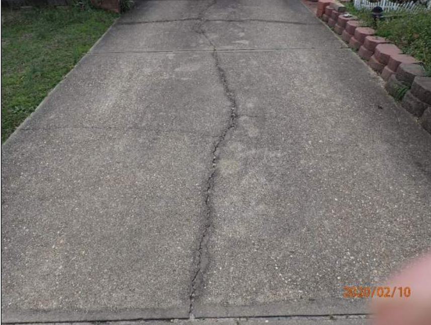
Photo 7 Cracks in concrete driveway
