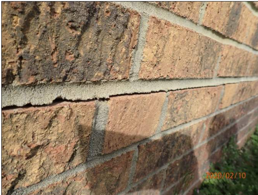
Photo 12 Horizontal crack (typical this elevation)
