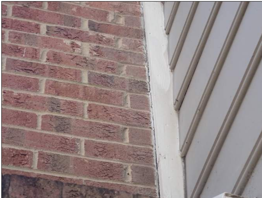
Photo 8 Chimney leaning outward
