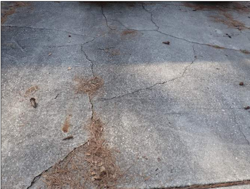
Photo 6 Cracks in concrete driveway
