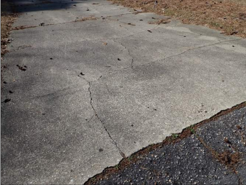
Photo 5 Cracks in concrete driveway
