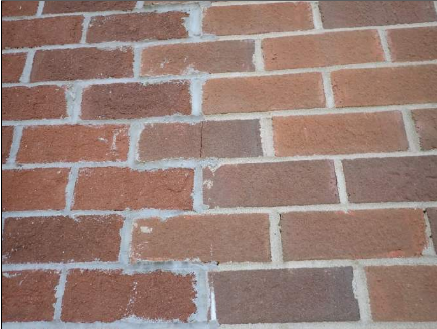
Photo 7 Individual cracked brick
