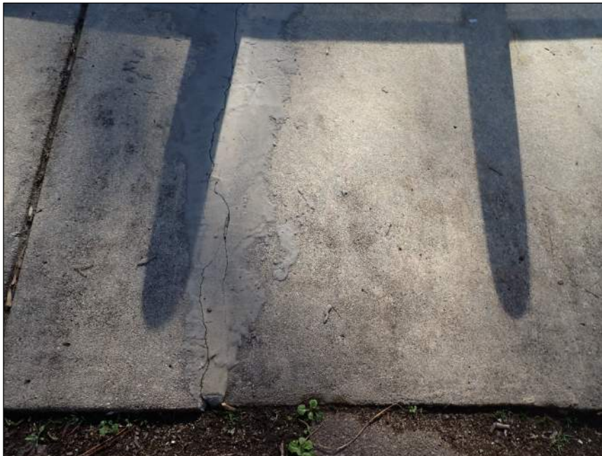
Photo 4 Cracks in concrete slab
