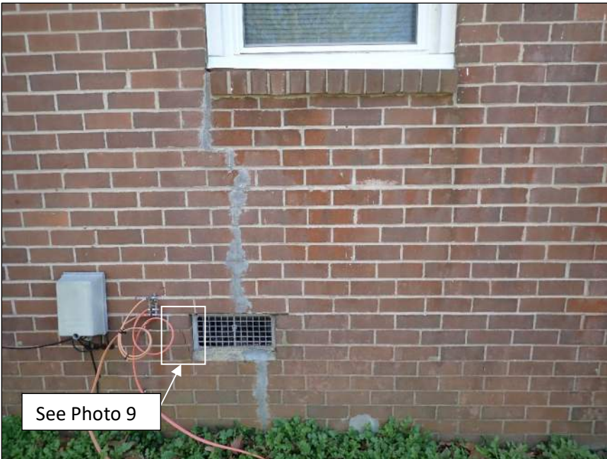
Photo 8 Previously repaired step crack
