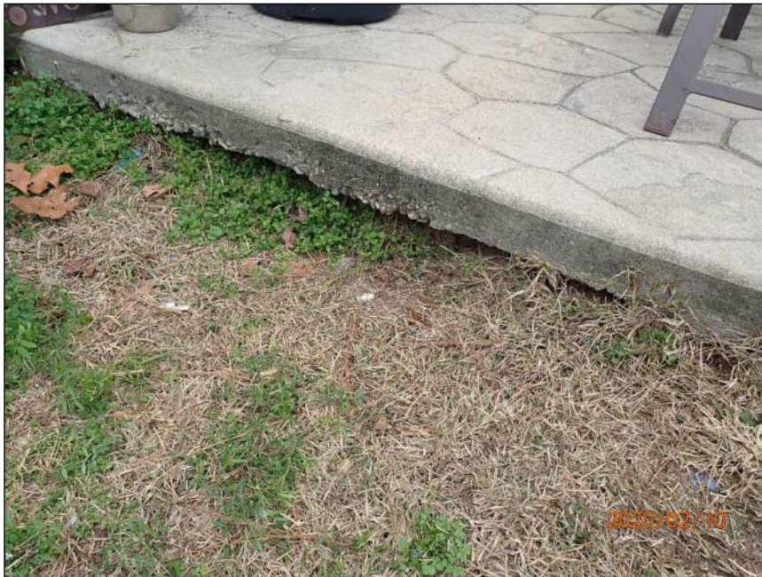
Photo 4 Undermined slab on grade
