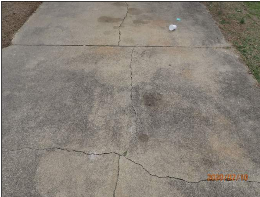
Photo 6 Cracks in concrete driveway
