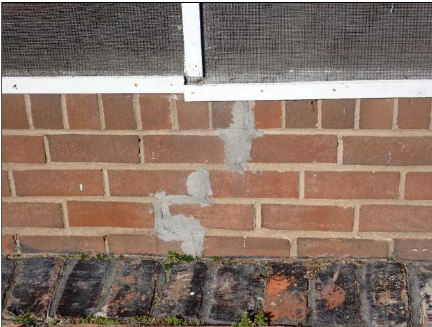
Photo 14 Previously repaired step crack
