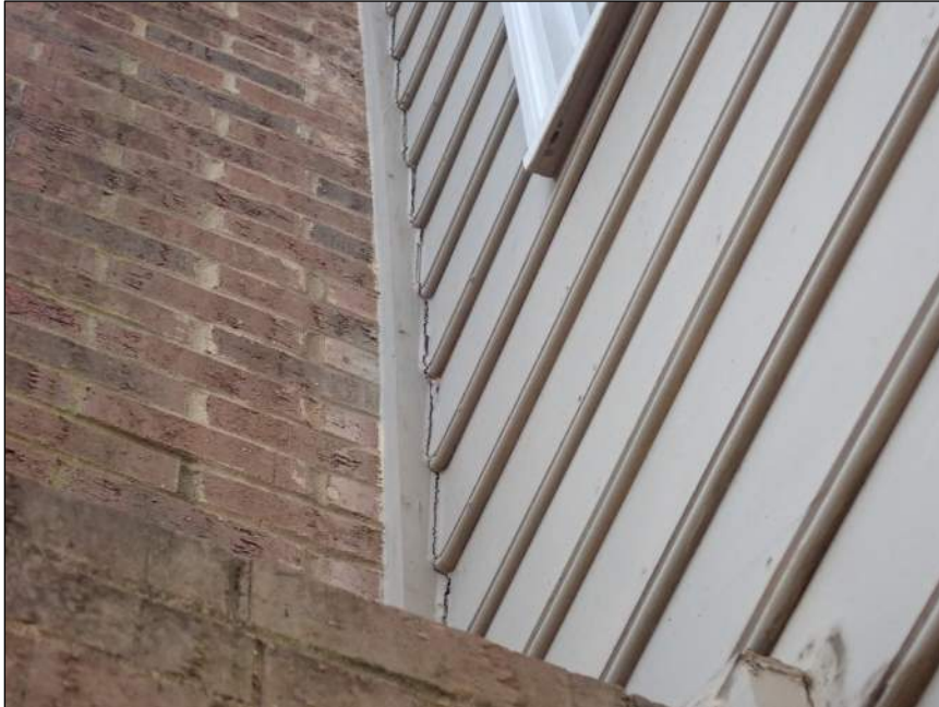
Photo 9 Chimney leaning outward
