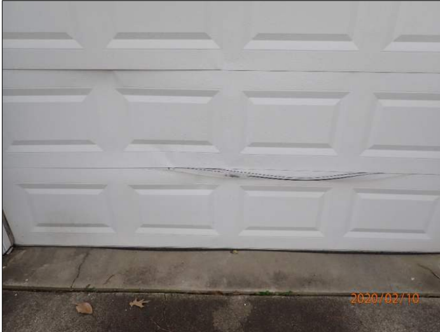
Photo 9 Damaged overhead garage door
