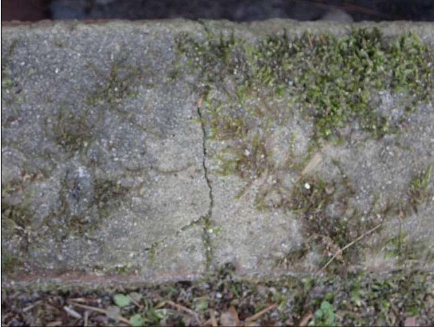
Photo 7 Crack in crawl space vent wells (typical)
