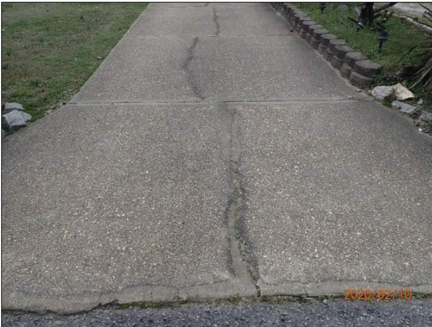
Photo 6 Cracks in concrete driveway
