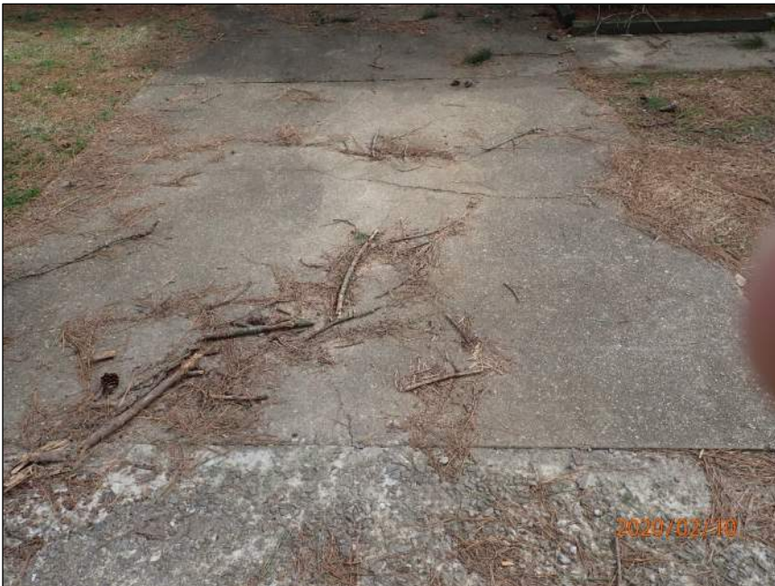
Photo 6 Cracks in concrete driveway
