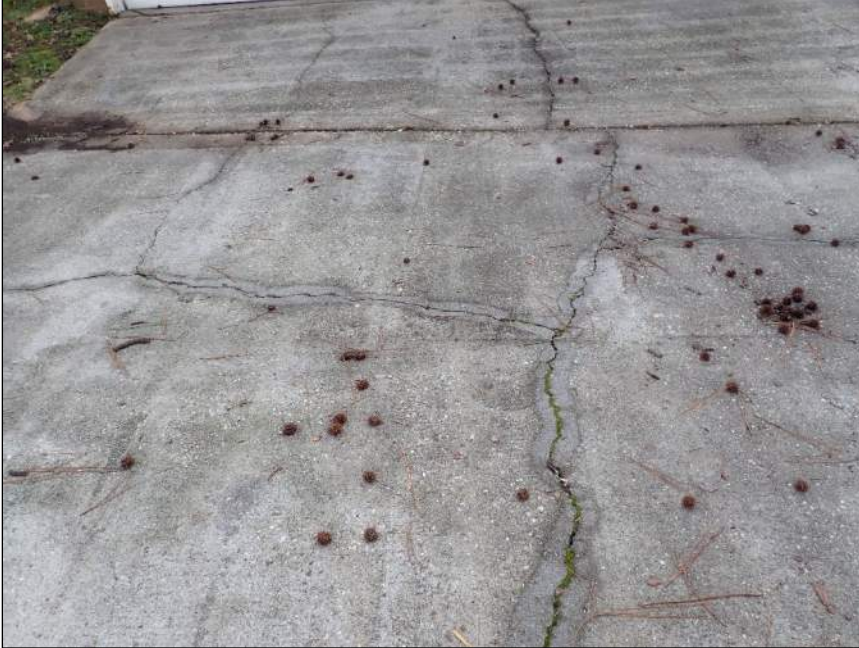
Photo 5 Cracks in concrete driveway
