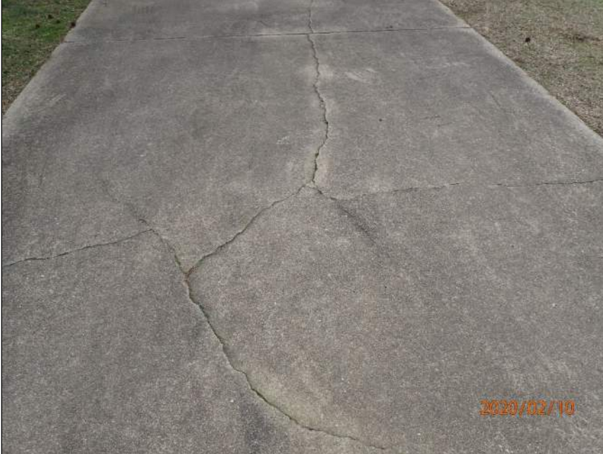
Photo 5 Cracks in concrete driveway
