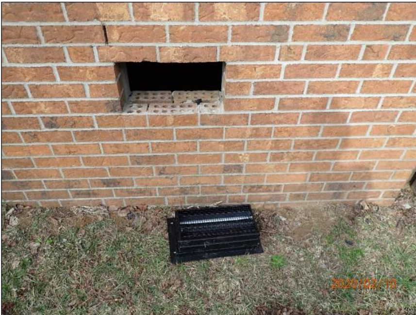
Photo 10 Displaced crawl space vents (typical)
