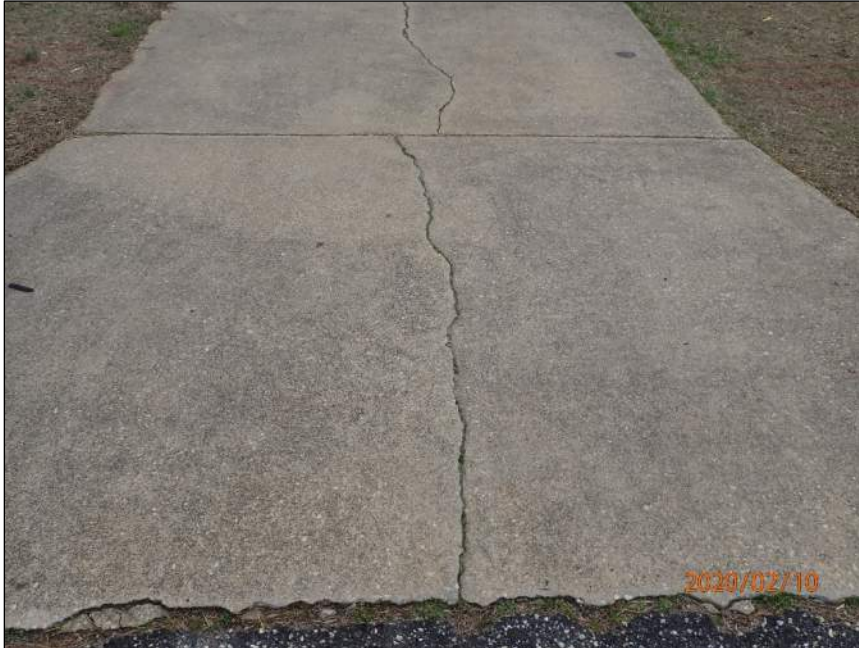
Photo 5 Cracks in concrete driveway
