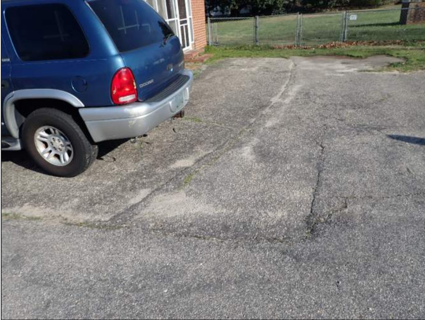
Photo 5 Cracks in driveway
