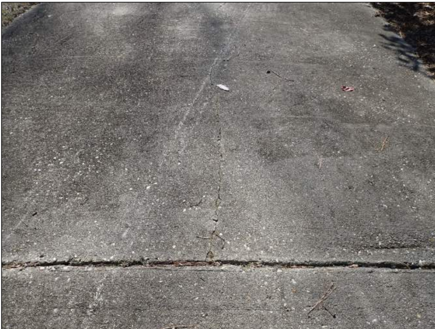
Photo 6 Cracks in concrete driveway
