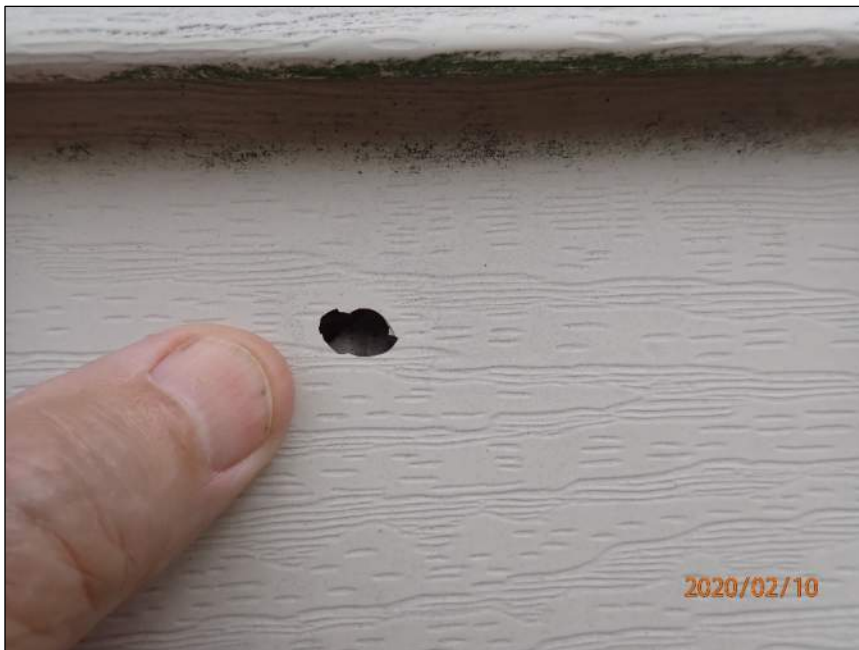
Photo 20 Hole in vinyl siding (typical)
