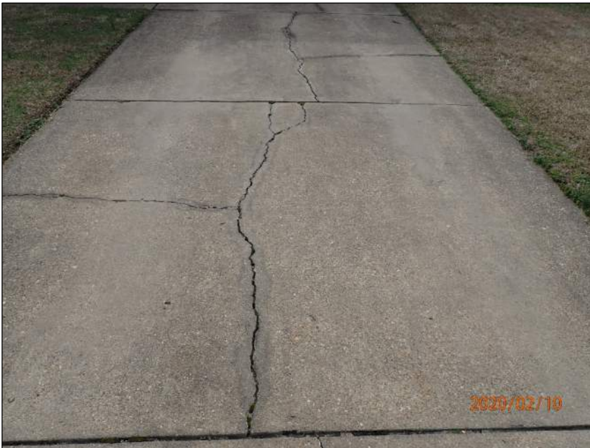
Photo 6 Cracks in concrete driveway
