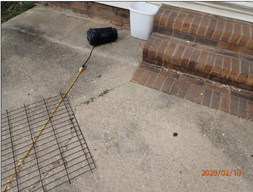
Photo 18 Cracks in concrete slab
