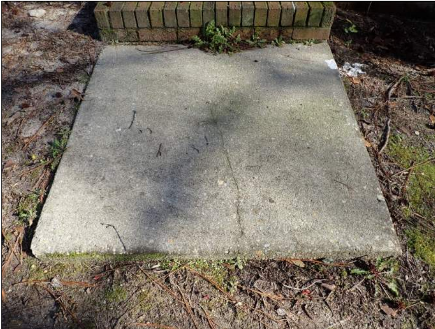
Photo 10 Cracks in concrete slab
