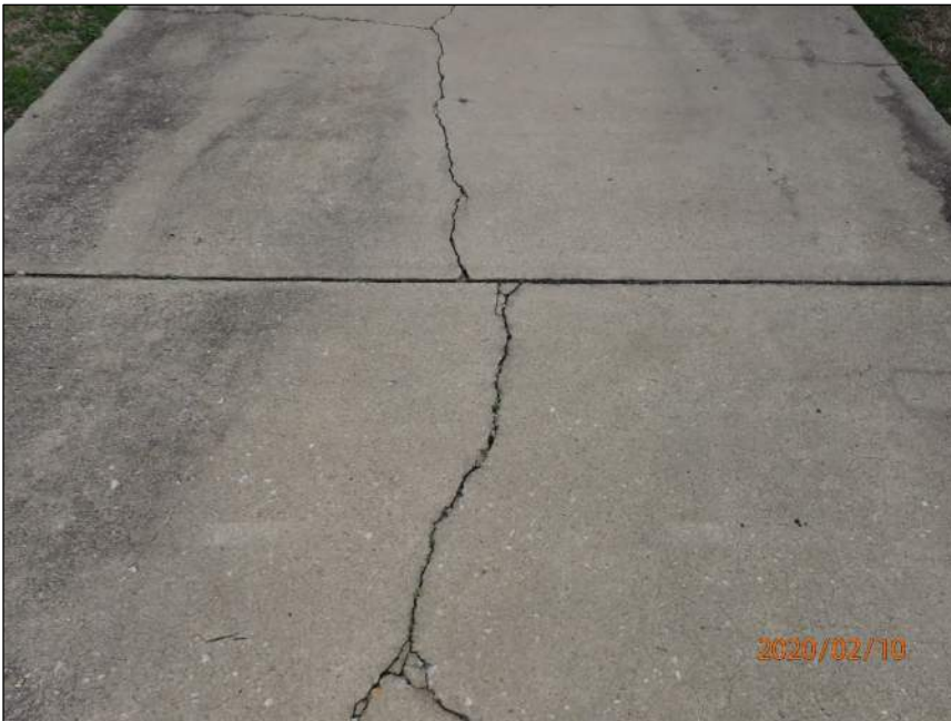
Photo 6 Cracks in concrete driveway
