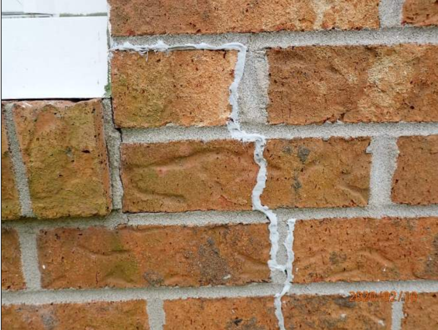
Photo 7 Previously repaired vertical crack
