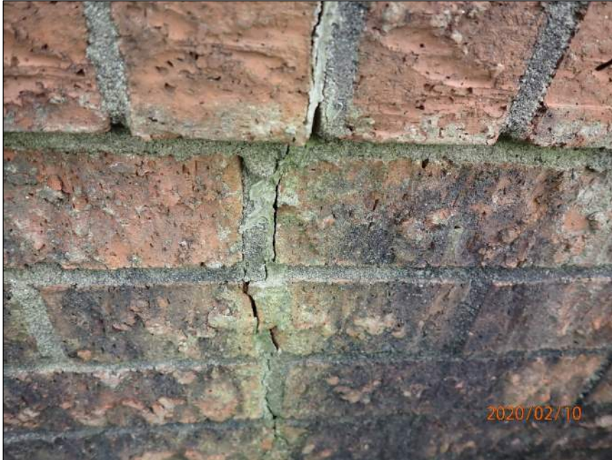
Photo 7 Previously repaired vertical crack
