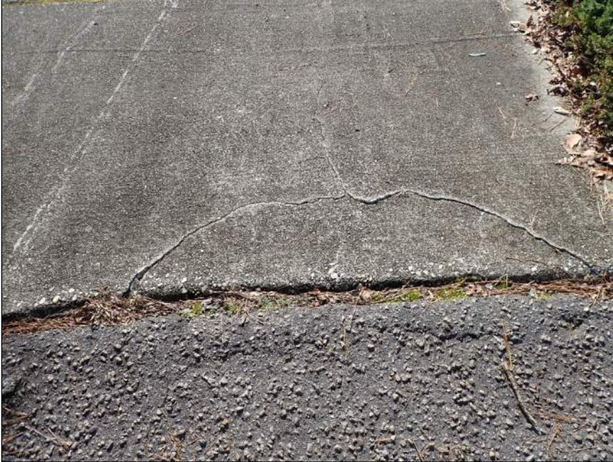
Photo 5 Cracks in concrete driveway
