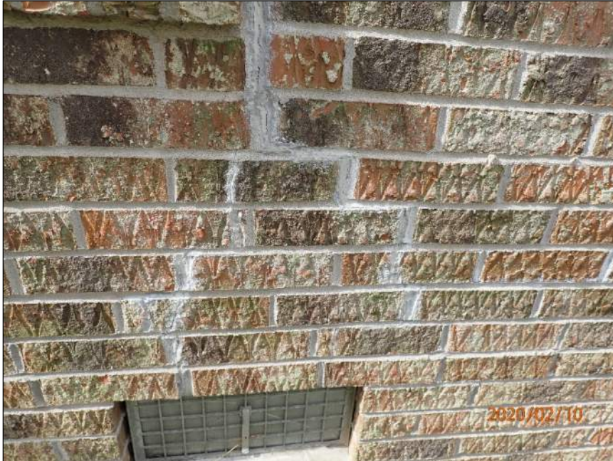
Photo 9 Previously repaired step crack
