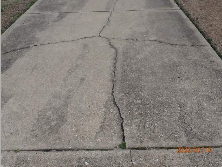
Photo 5 Cracks in concrete driveway
