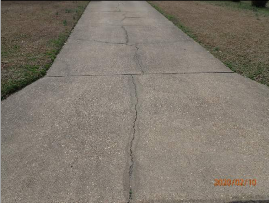
Photo 5 Cracks in concrete driveway
