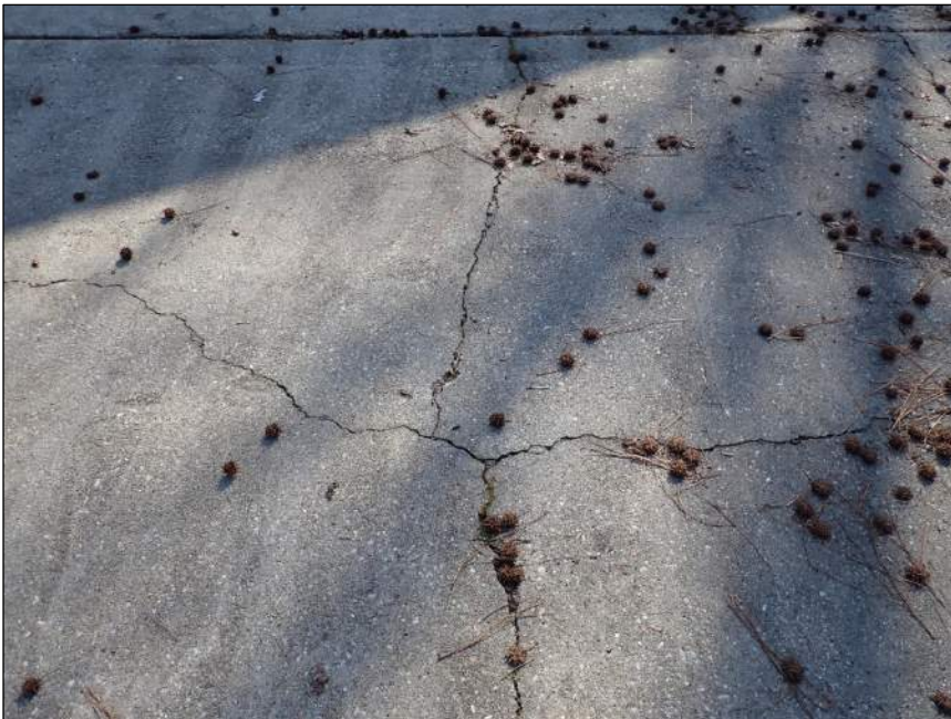
Photo 6 Cracks in concrete driveway
