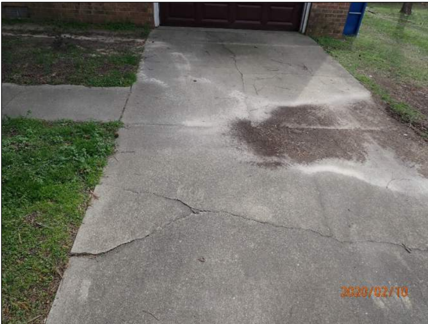
Photo 6 Cracks in concrete driveway
