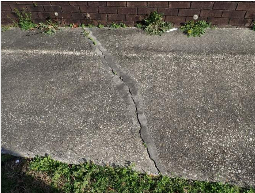
Photo 6 Cracks in concrete slab
