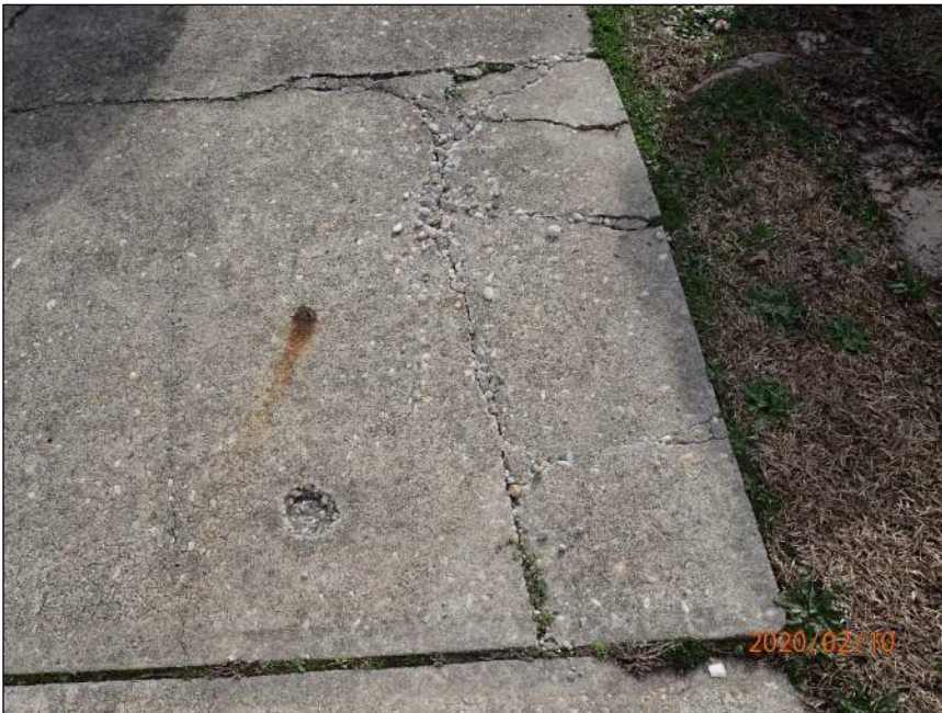
Photo 6 Cracks in concrete driveway
