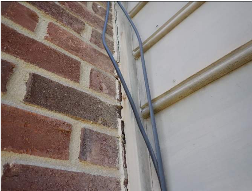
Photo 8 Chimney leaning outward
