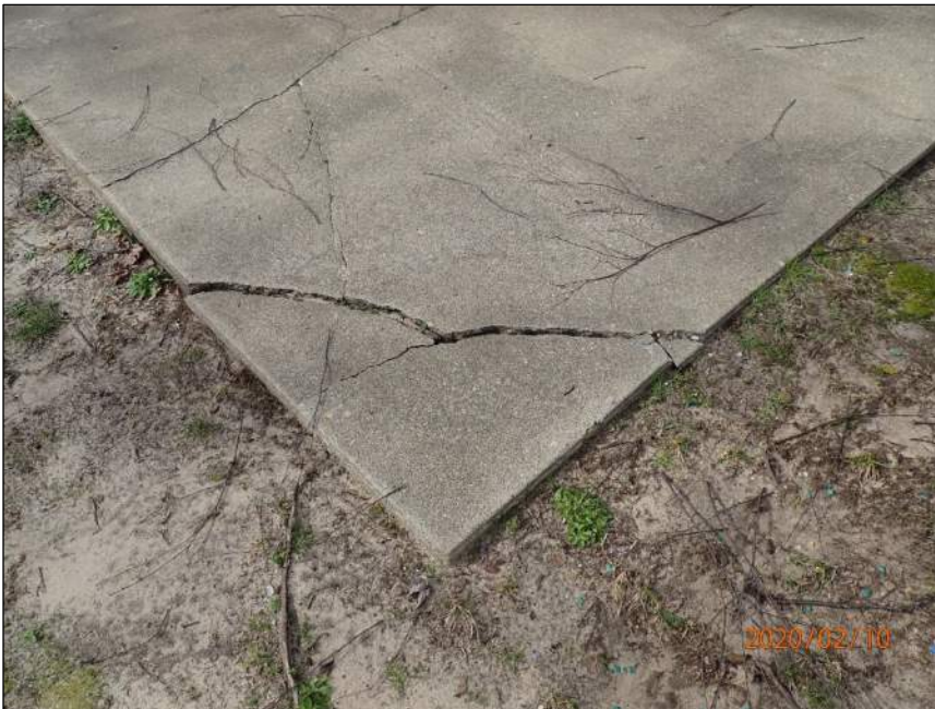
Photo 16 Cracks in concrete slab
