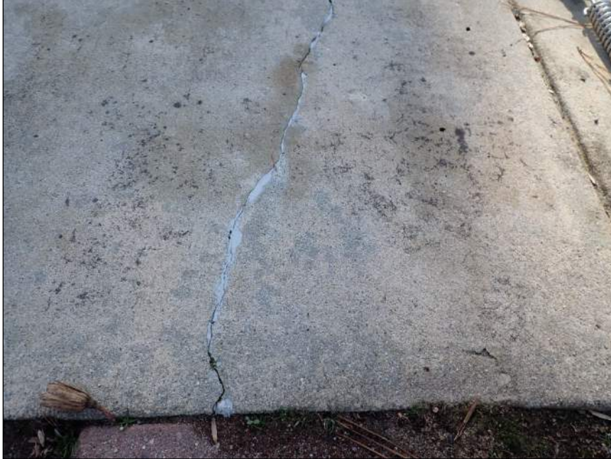
Photo 5 Previously repaired cracks in concrete slab
