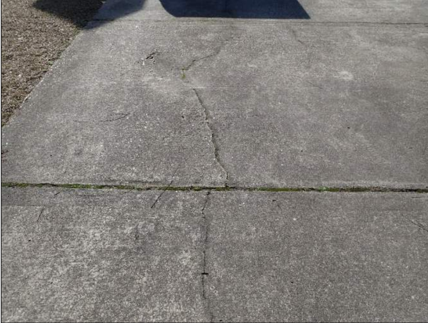
Photo 5 Cracks in concrete driveway
